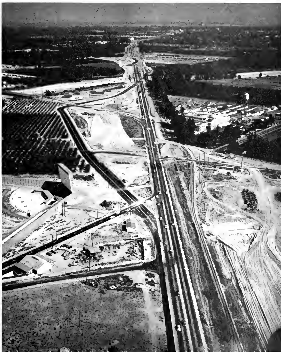
Looking southeasterly along construction in progress on Santa Ana Freeway with the site of the Chapman Avenue Traffic Interchange System shown in center. Orange County Hospital buildings are shown center right.
